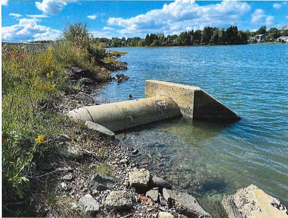
Photo 1 – Existing outfall headwall, exposed 48” RCP pipe, and tidal embankment looking west at high tide. Taken 9/28/22
