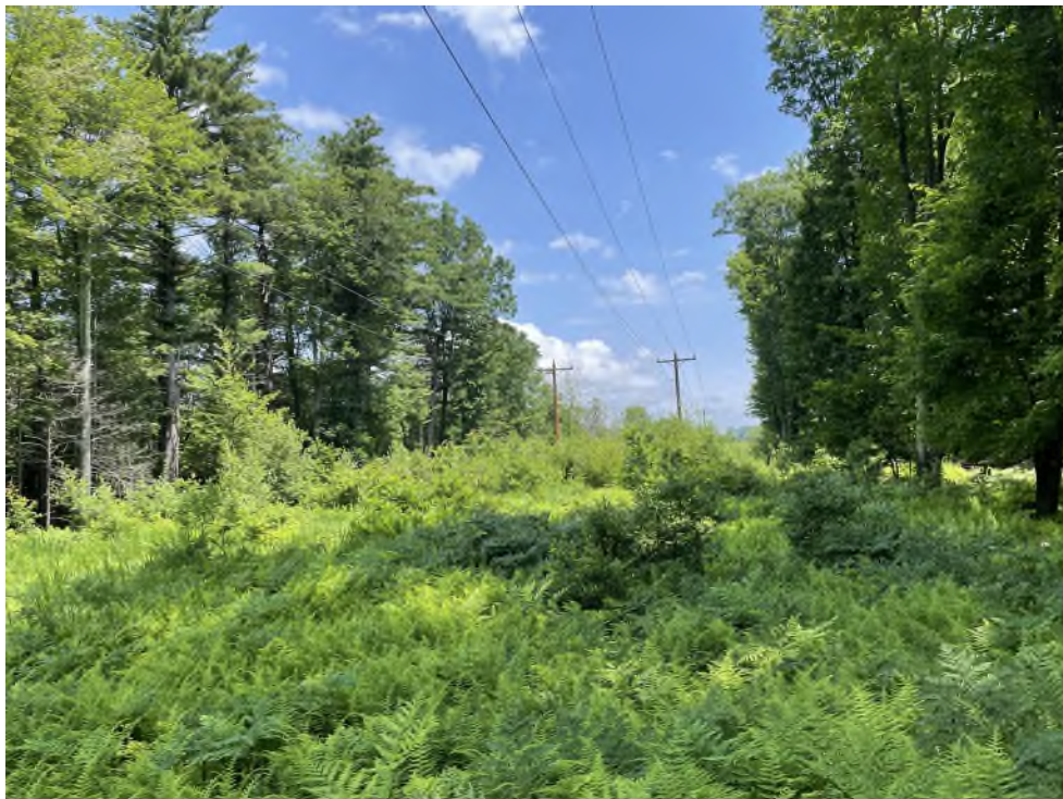
Photograph No. 8: Looking north towards Structure 86 on the 3171 Line ROW off Ocean Road, Portsmouth, NH.
