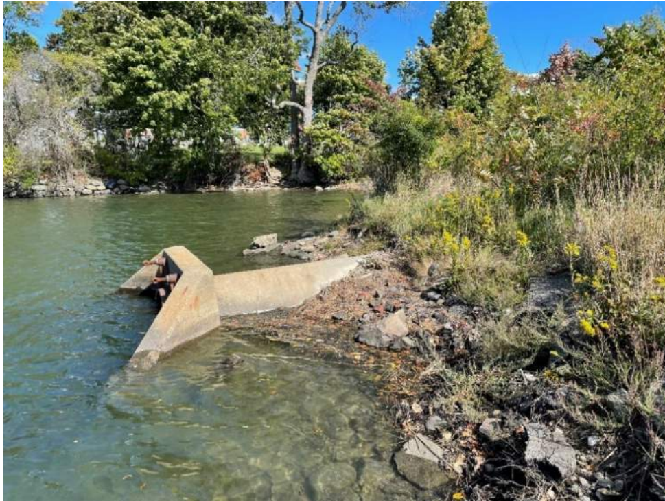
Photo 3 – Existing outfall headwall, exposed 48” RCP pipe, and tidal embankment looking east at approximate high tide. Taken 9/28/22
