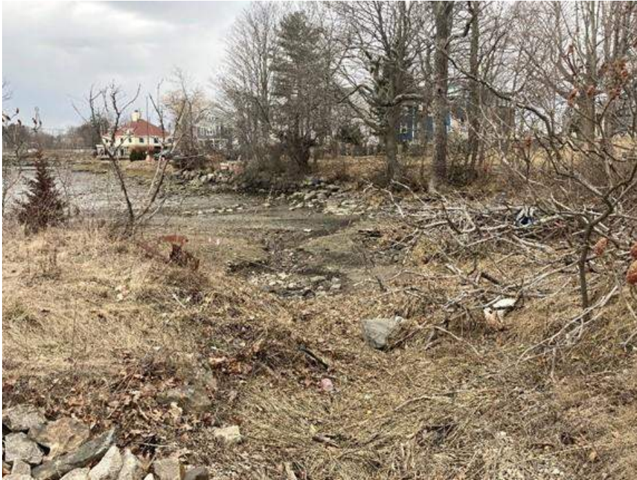
Photo 15 – Existing drainage swale outlet (to be eliminated) and erosion in mitigation area looking north at approximate low tide. Taken 3/20/24
