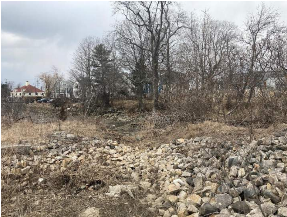
Photo 16 – Existing drainage swale (to be eliminated) looking north at approximate low tide. Taken 3/20/24
