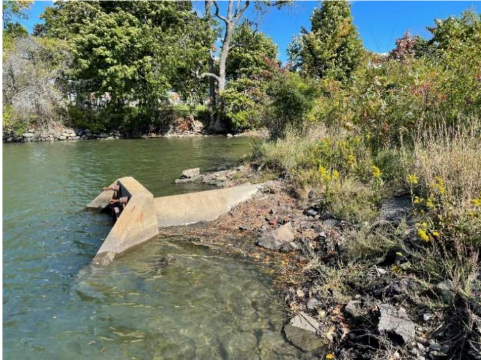
Photo 3 – Existing outfall headwall, exposed 48” RCP pipe, and tidal embankment looking east at approximate high tide. Taken 9/28/22
