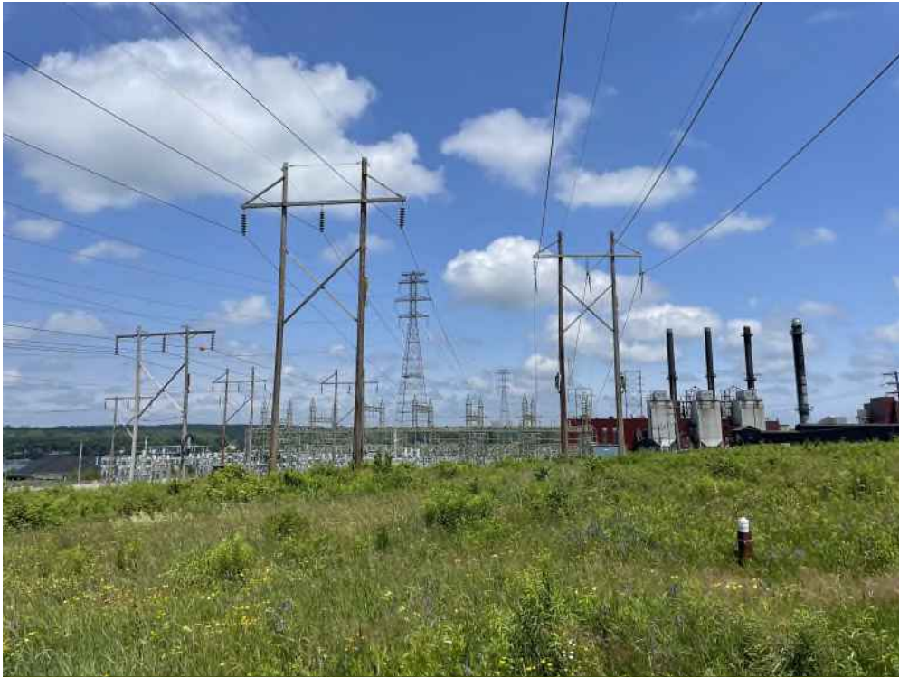
Photograph No. 19: Looking northeast at Structure 1 on the T13 Line ROW off Gosling Road, Portsmouth, NH.
