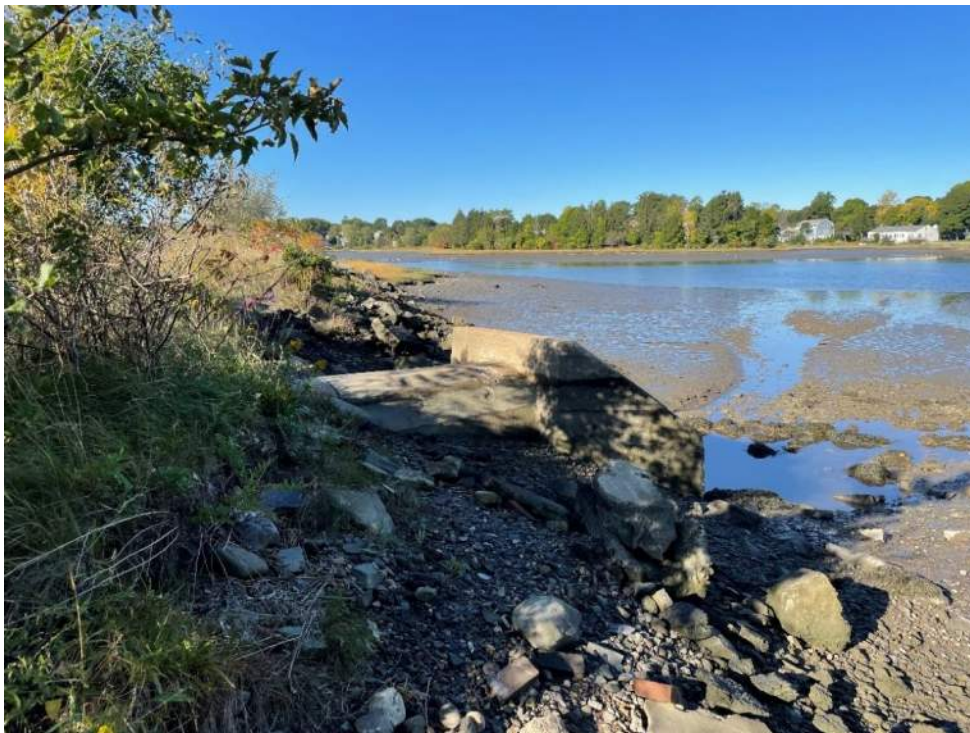
Photo 4 – Existing outfall headwall, exposed 48” RCP pipe, and tidal embankment looking west at approximate low tide. Taken 9/29/22
