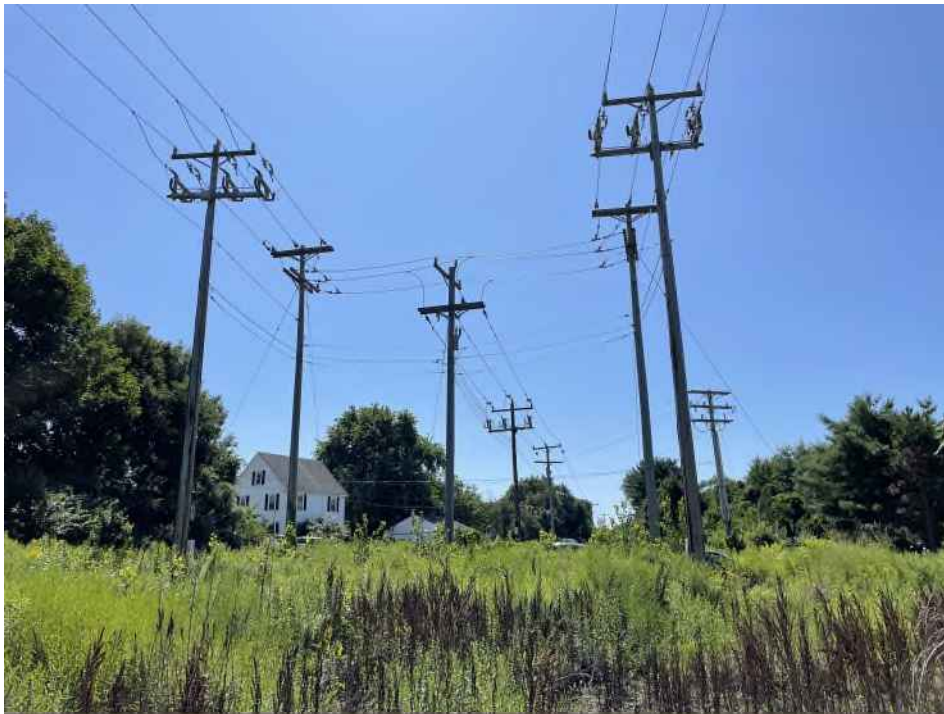
Photograph No. 18: Looking southeast at Structures 72.1 to 72.5 on the 3171 Line ROW off Griffin Road, Portsmouth, NH.
