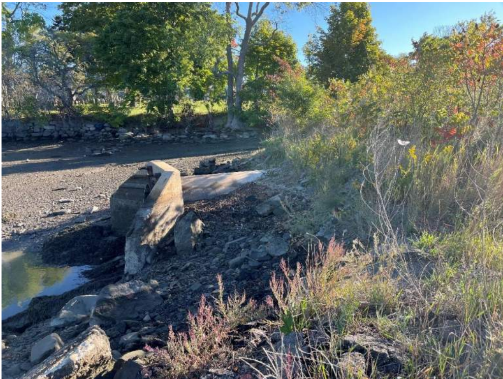
Photo 6 – Existing outfall headwall, exposed 48” RCP pipe, and tidal embankment looking east at approximate low tide. Taken 9/29/22
