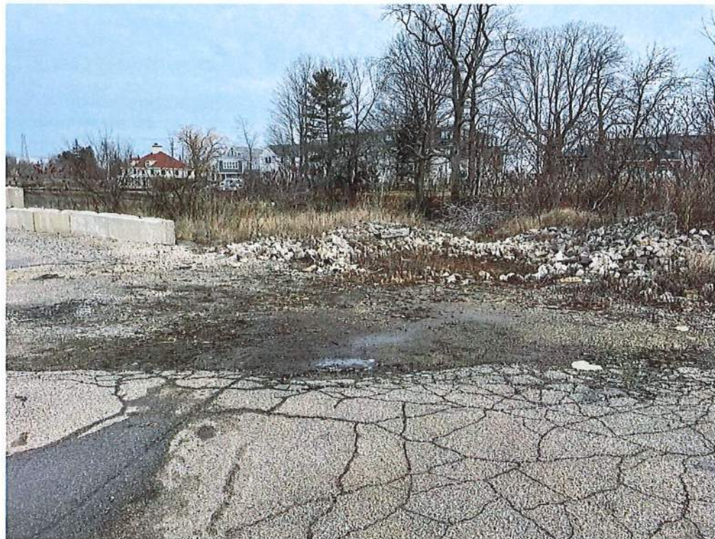
Photo 4 – Edge of 90 Maplewood Ave LLC lot looking north with existing pipe located parallel to concrete block wall flowing west to outfall. Taken 1/19/23
