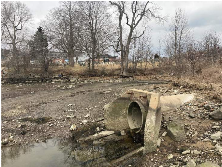
Photo 12 – Existing outfall headwall with mitigation area in background looking east at approximate low tide. Taken 3/20/24
