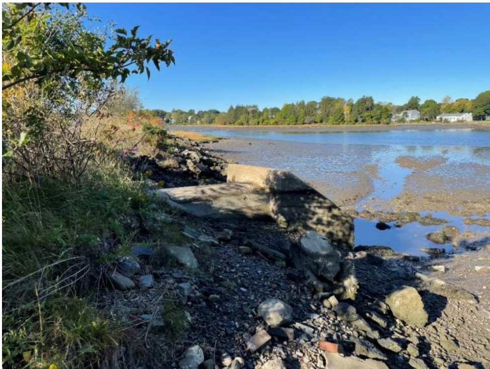
Photo 4 – Existing outfall headwall, exposed 48” RCP pipe, and tidal embankment looking west at approximate low tide. Taken 9/29/22
